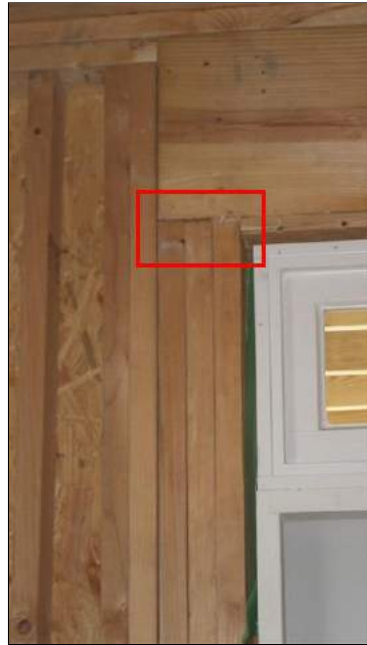
(3) Header-to-stud framing was not done tightly at the front door at the left side.
