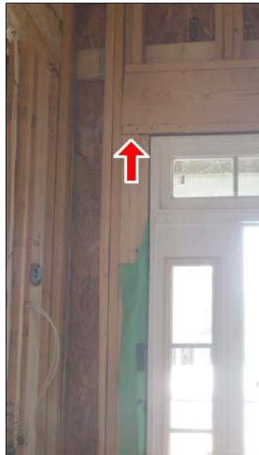
(4) Inside the master bedroom at the family room wall, the bottom of one of the studs is damaged.
