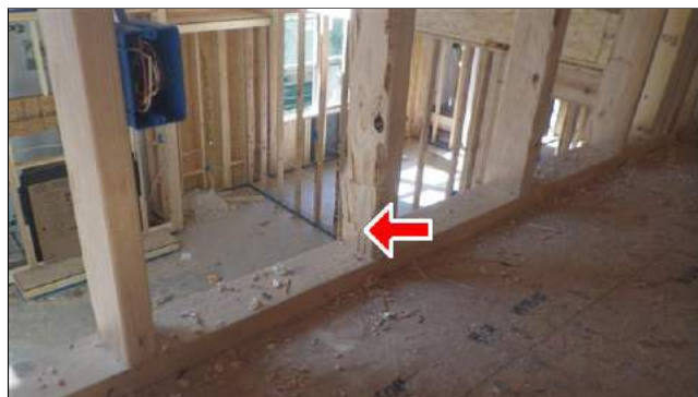
(5) A bowed stud was observed in the master bathroom next to the smaller window.
